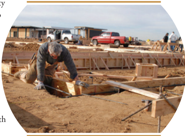
HIGH SCHOOL — Worker building forms for foundations at the new California City High School. BILL DEAVER/Desert News
